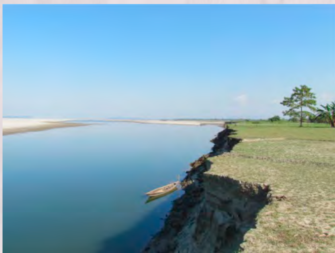
Erosion on the bank of River Brahmaputra Tezpur, Assam
