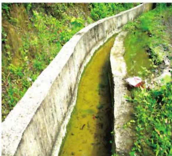
Rain water drainage on Laxmi Nagar
