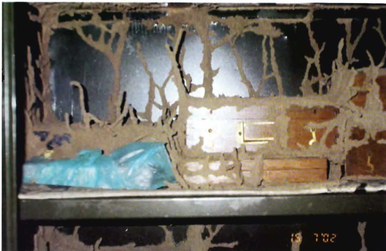
5. Damage caused by Microtermes mycophagus to wooden boxes and paper register (Jodhpur district)
