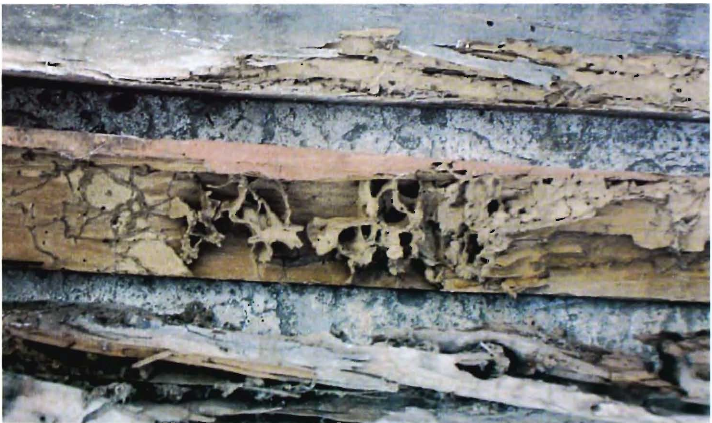
20. Wooden door frame damaged by Coptotermes heimi (Jodhpur district)
